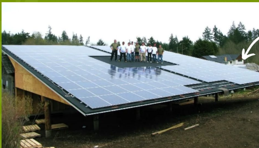
Part of the solar array at T'Sou-ke First Nation
